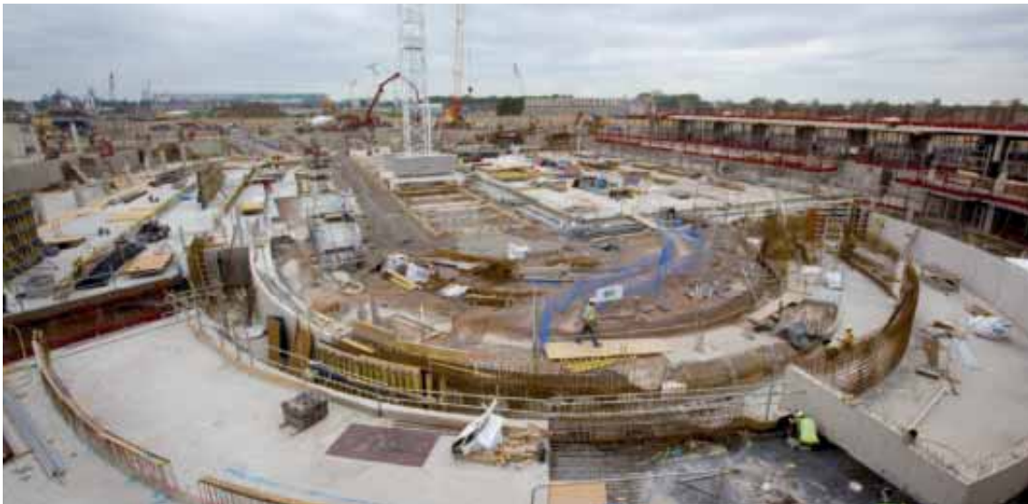
Velodrome taking shape in August 2009. The Velodrome design is lightweight and achieves a 44 per cent reduction in potable water against industry standards and 36 per cent reduction in energy use against Part L 2006 Building Regulations.
